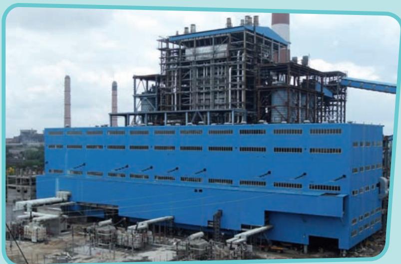
Khaparkheda Thermal Power Station 1x500 MW BoP MAHAGENCO, Nagpur Maharashtra | March 2011
