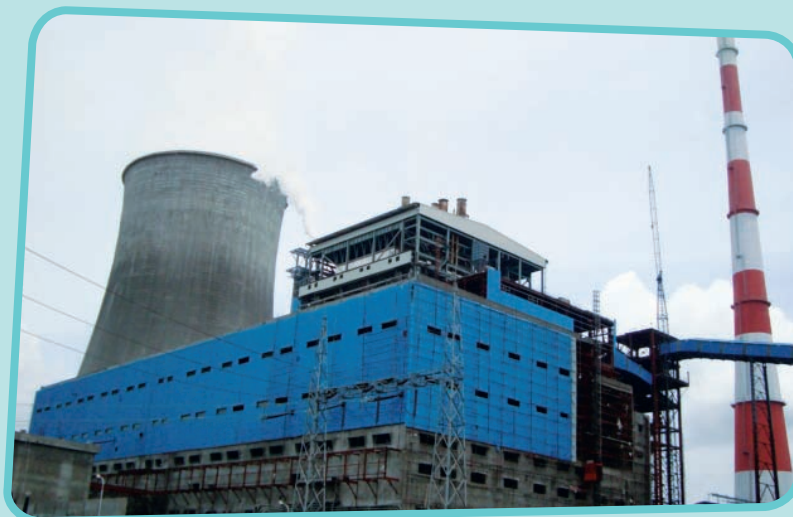
Kothagudem Thermal Power Station 1x500 MW BoP APGENCO, Khammam Andhra Pradesh | March 2011
